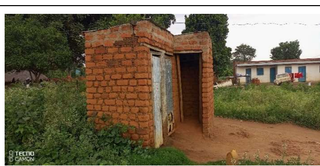
Dilapidated latrine at the Goboro Market
