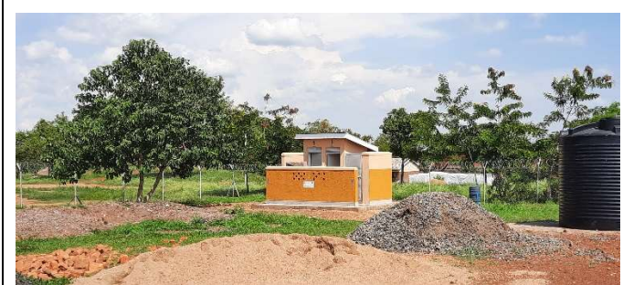
VIP toilet at UNHCR Refugees Reception Centre
