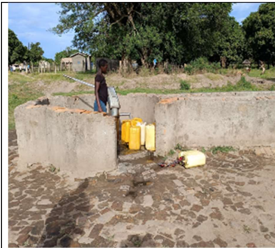
Figure 6-13: Borehole for the Community at Idijo Village
