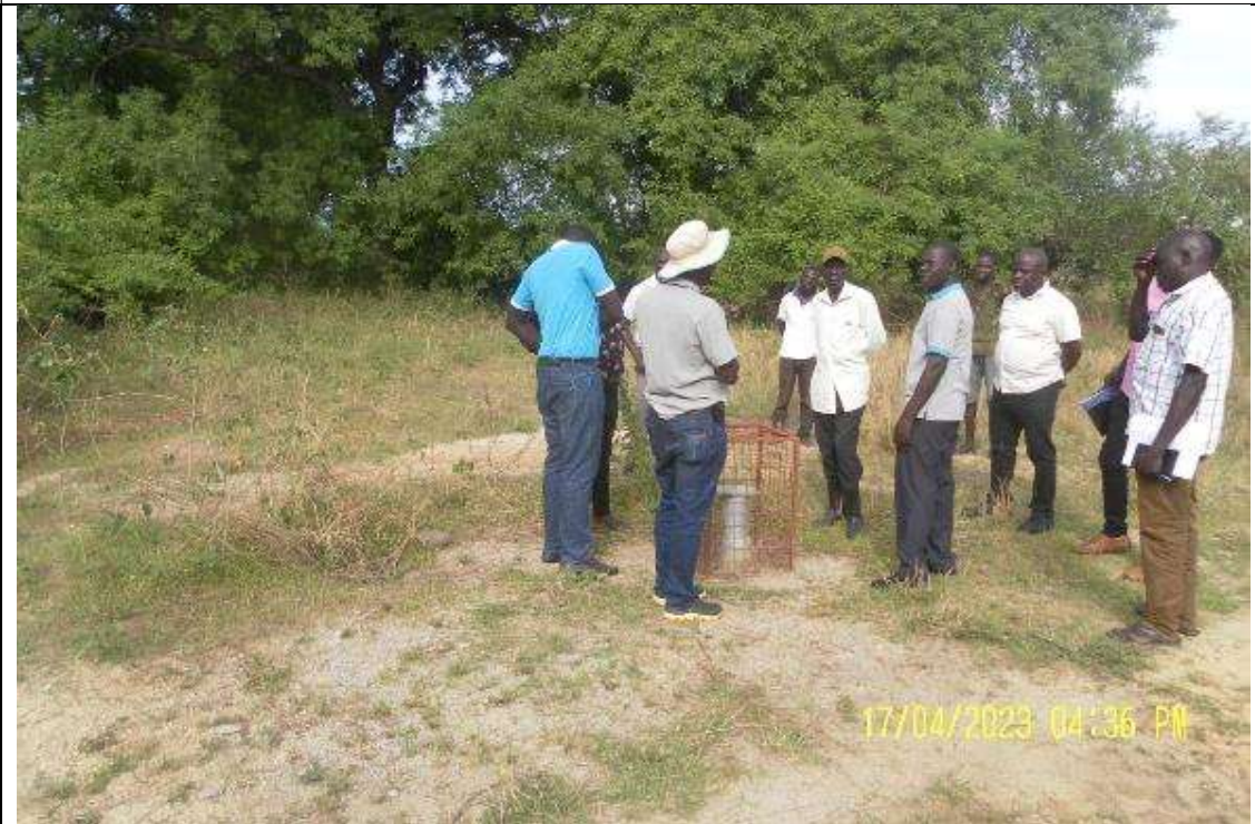
MWE staff, Consultant and Laropi Town Council staff Inspecting the Proposed Production well for Laropi RGC
