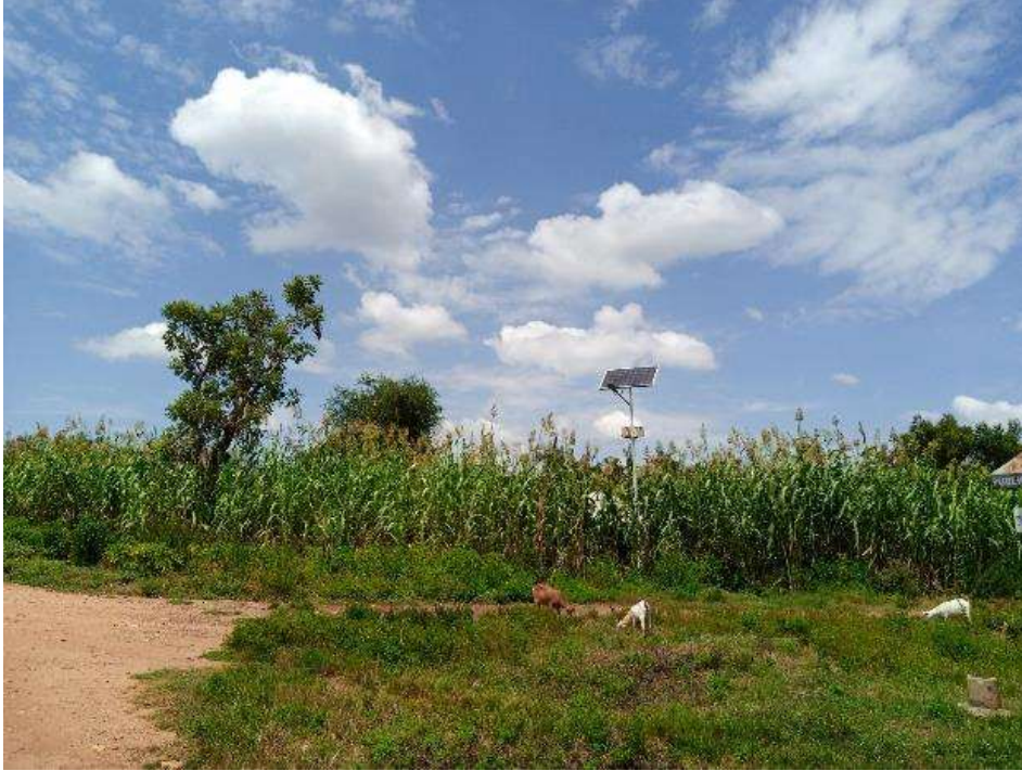
Plate 5.15: One of the public solar lighting systems
