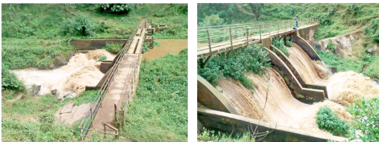
Figure 4-25: Silt and Vegetation growth at Maziba mini hydropower dam
