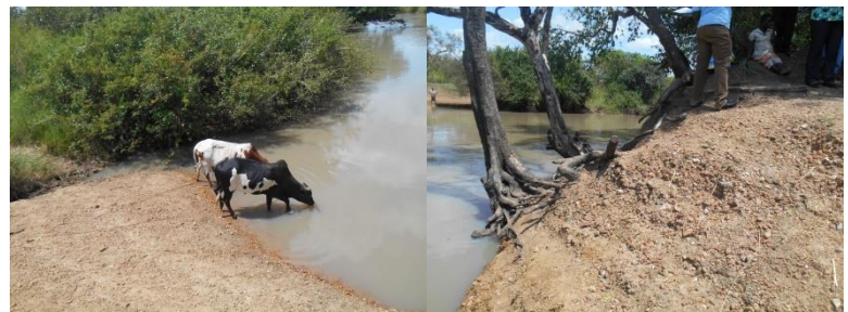
Figure 1-7: Collapsing of river banks due to uncontrolled access of livestock to River Aswa in Angole A Village, Aromo subcounty, Lira District
