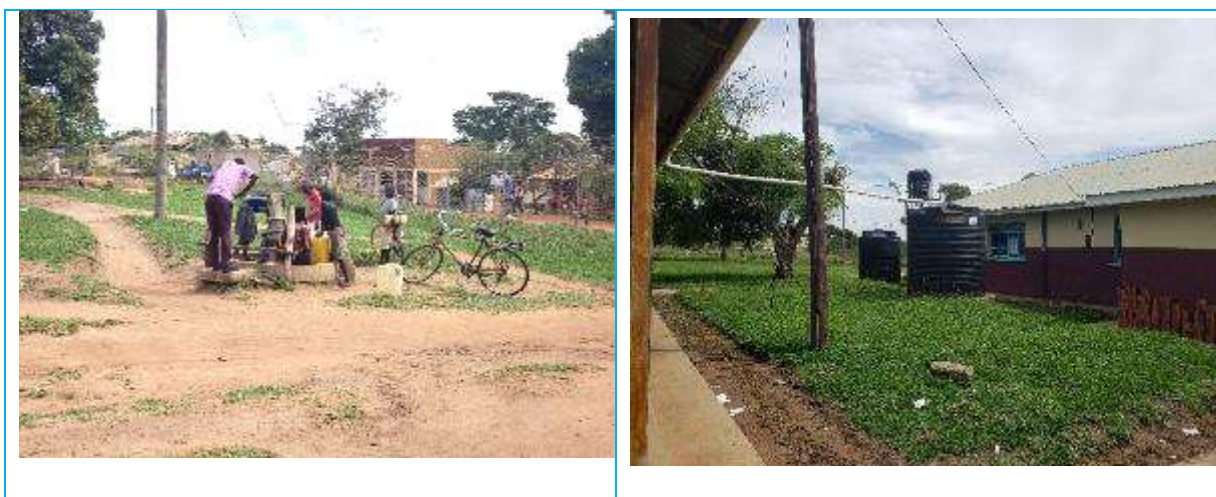
Figure 6-39: Deep borehole and RWHT at Kidera HC IV in Kidera RGC
