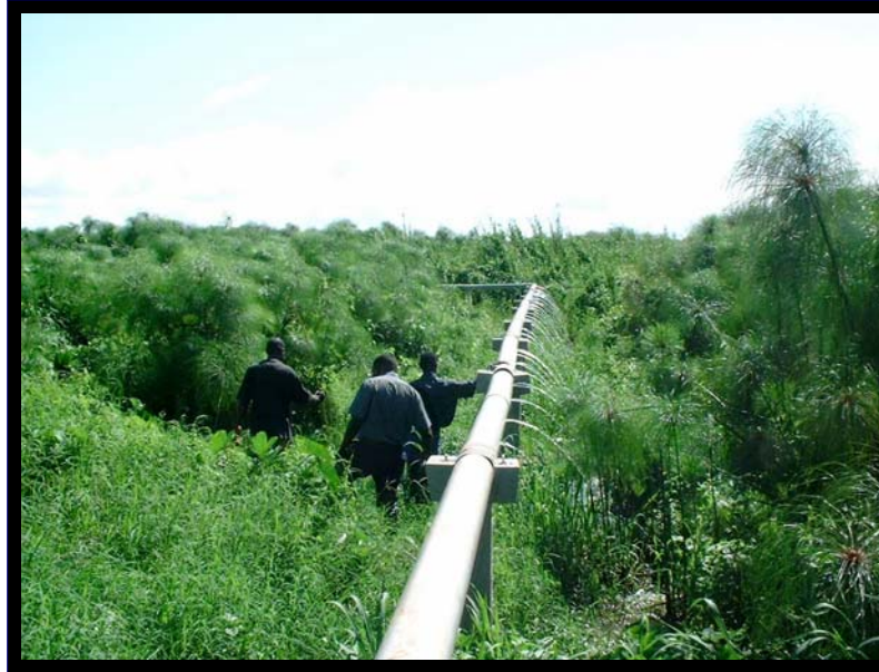
FIG. 2. Wastewater distribution pipe at the edge of the wetland
