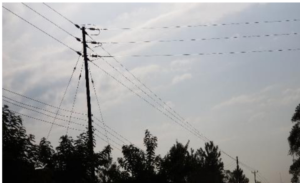
Plate 11: A hydroelectricity transmission line in Kirewa Sub-county. Photo taken by the Sociologist on 11 th March 2023
