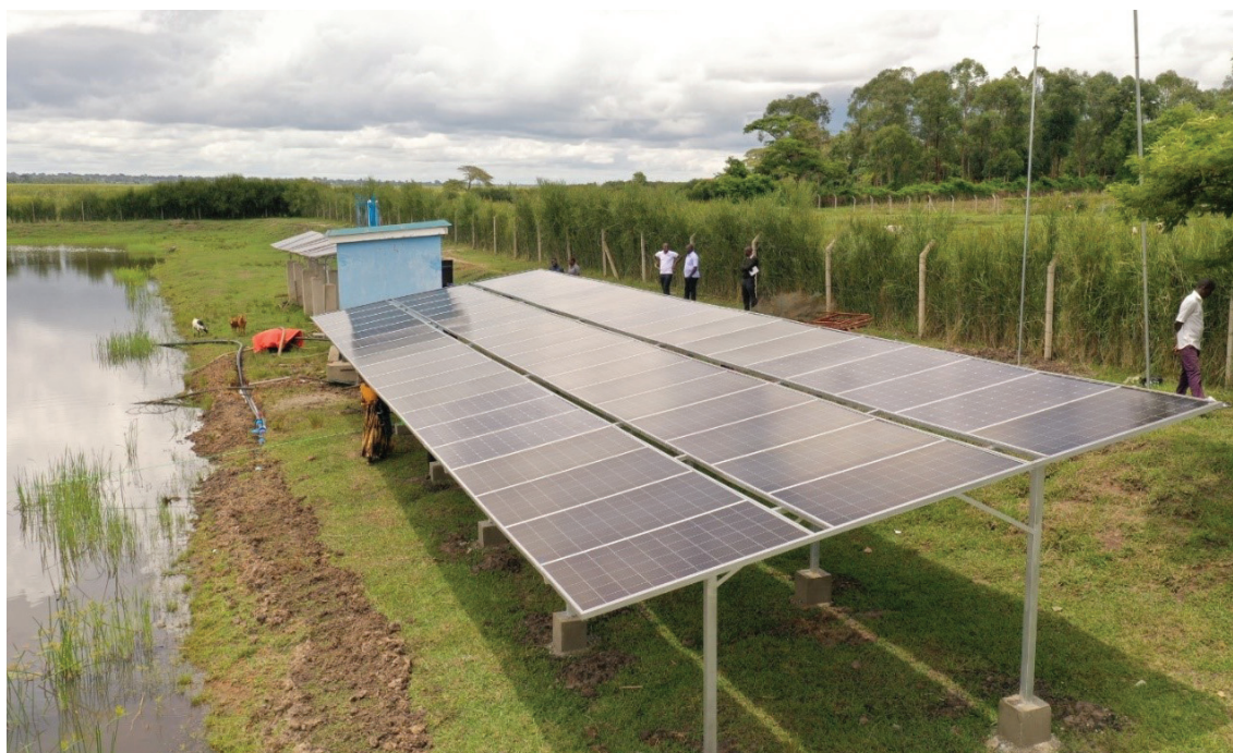
Solar panels at Limoto small scale irrigation scheme
