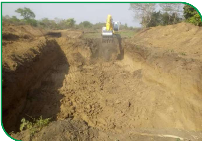
Excavation of the river diversion channel at Wadelai irrigation scheme, Pakwach district ■
