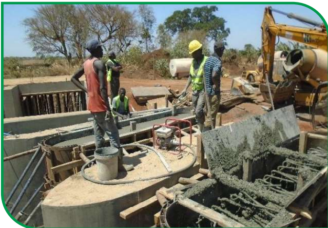
Concrete casting of piers at intake one at river Kabajiria, Ngenge irrigation scheme, Kween district ■
