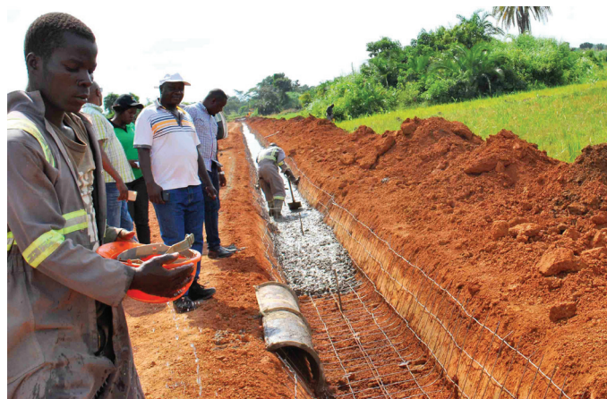
Some of the workers carrying out rehabilitation works at one of the canals of Olwenyi irrigation scheme in Lira district
