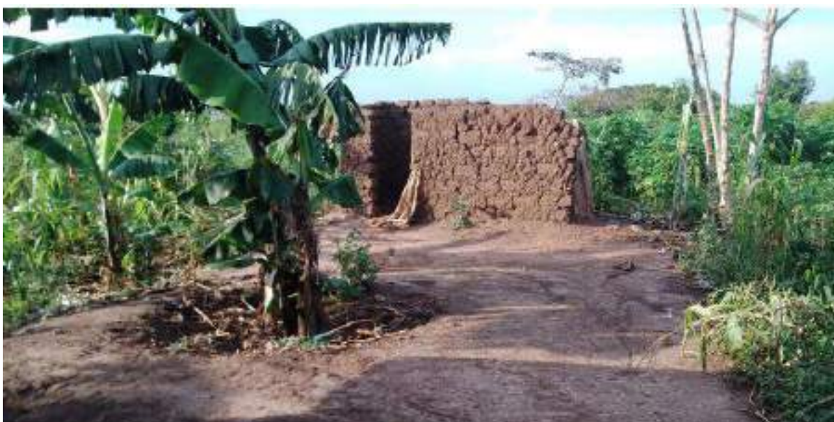
Figure 0-73: Poor pit latrine in Mutunda RGC
