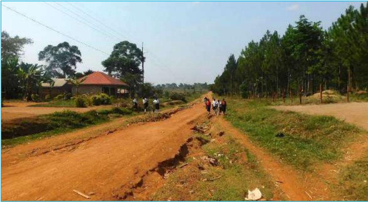
Figure 6-20: Narrow section of the Kaliro-Nawaikoike-Buvuluguti Road with gullies in Lwamba TC
