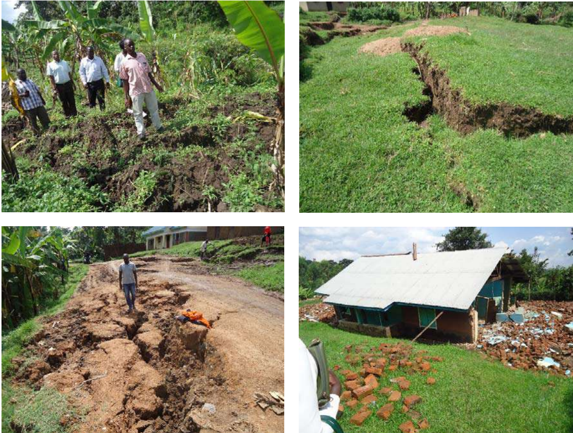
Figure 8.1 - SMEC and the District team inspect an area affected by land slides and land cracking in the Namisindwa District (source: SMEC, 2018)
