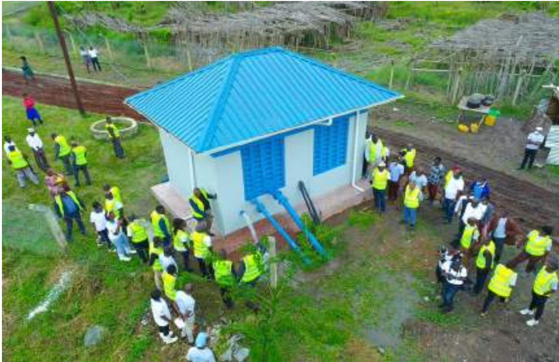
WSDF-Central staff together with Kagadi stakeholders inspecting the wash out at the pump house for Kagadi Piped Water Supply System.
