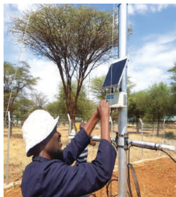
Weather Station at Rupa, Moroto
