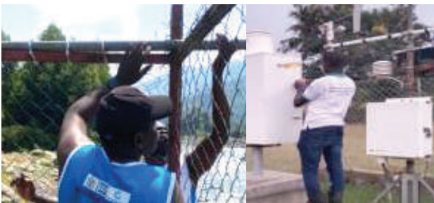
Figure shows automatic station installed in Kasese and water level sensor installed in River Mubuku
