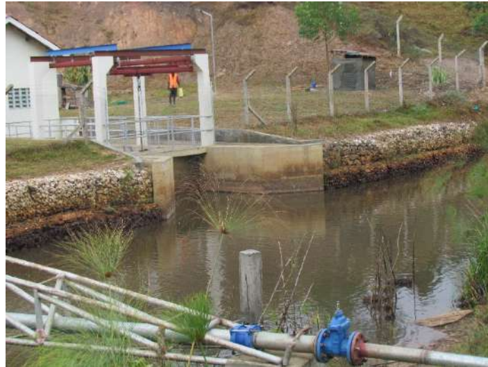
Plate 47: Water pumping and treatment station in Sheema District
