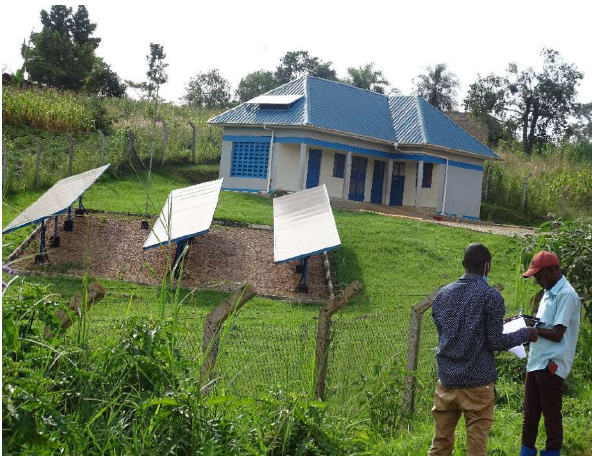
Plate 9: Kabwoya-Kyakatwanga-Nyamarwa water supply system in Nyamambukabiri wetland in Kibaale district
