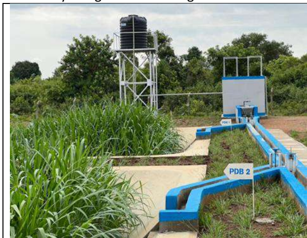
Photo 1: Mixing and grit chamber for separation of solids from liquids at Yumbe FSTP
