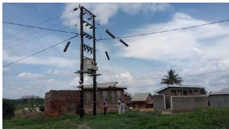
Picture 2.5: Transformer within Lugala Center
