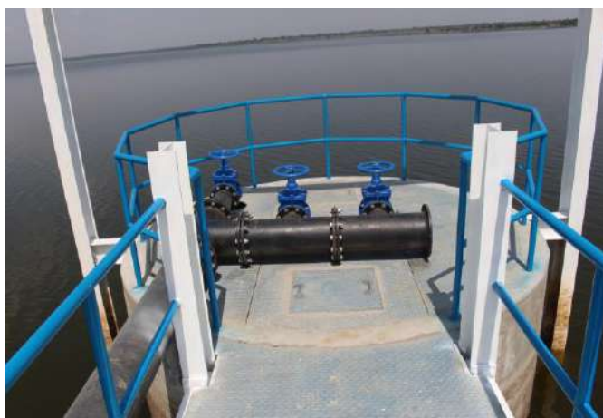
Picture 4.1: Intake Structure with raw water pipe on side of access bridge.
