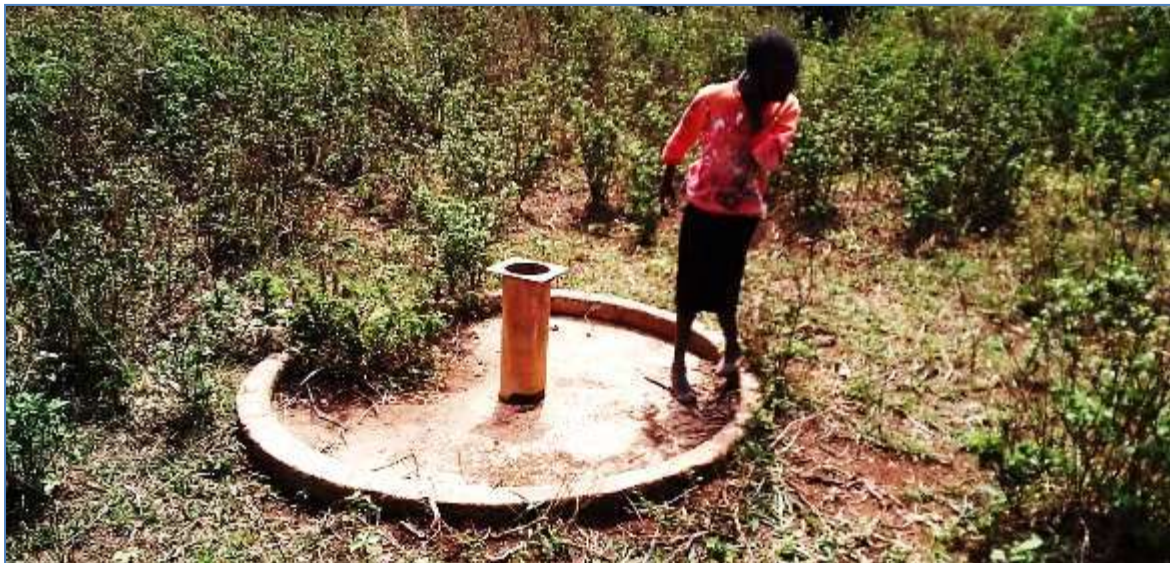
Figure 6-55: Abandoned deep borehole at Nabuuku village in Igwaya RGC
