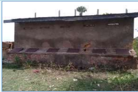
Damaged public latrine at Buyumba landing site
