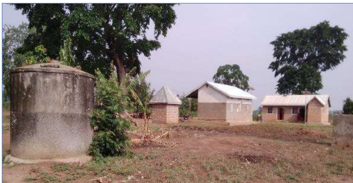
Figure 6-64: Damaged concrete water tank at Kagulu HC III
