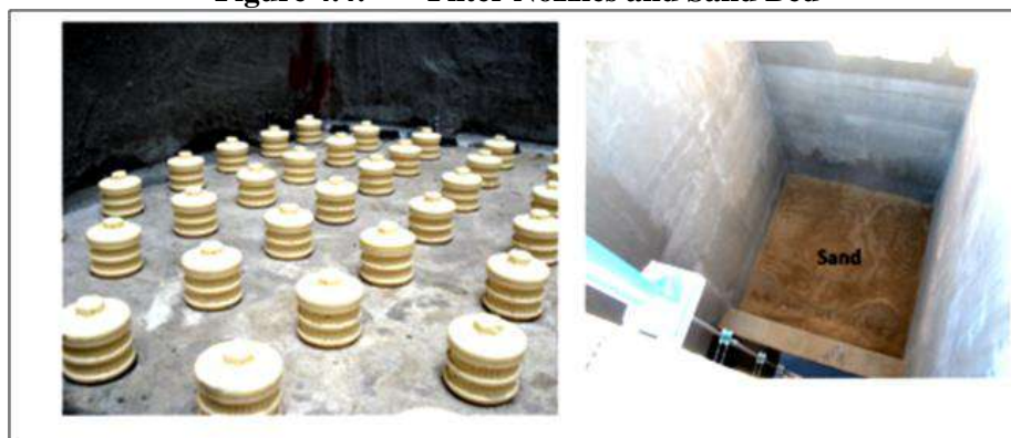
Figure 4.4: Filter Nozzles and Sand Bed
