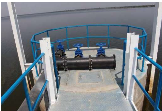
Picture 4.1: Intake Structure with raw water pipe on side of access bridge.
