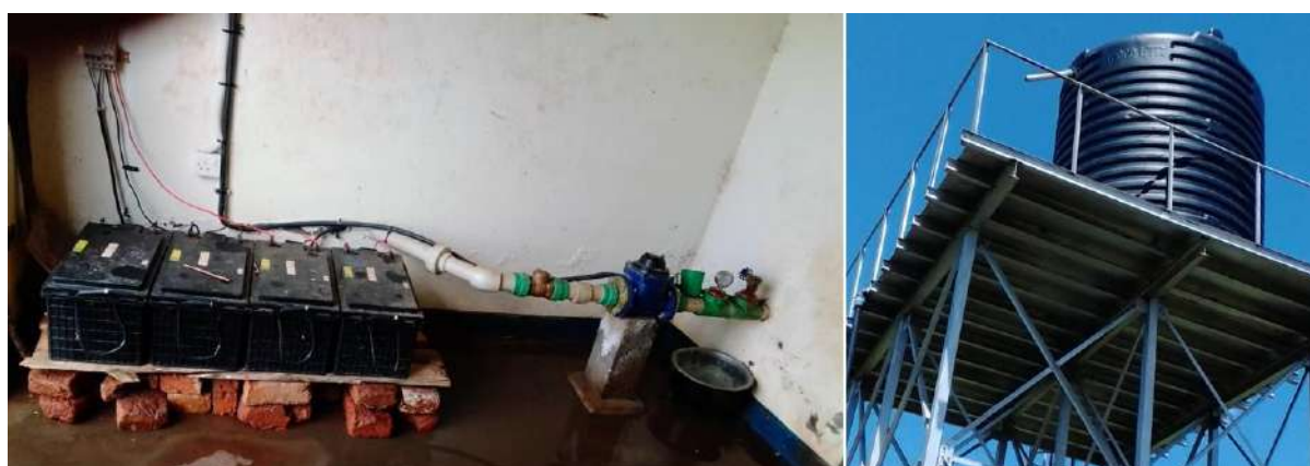
Figure 5-63: Current state of storage batteries and reservoir
