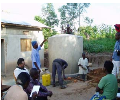
Communal RWH tank in Sheema, Bushenyi
